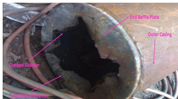
Figure No. 1 Actual cracked silencer end
