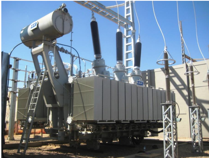
Figure 1. The magnetic part of the control shunt reactor transformer
