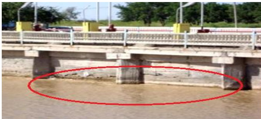
Figure 2. The regulation structure damages
