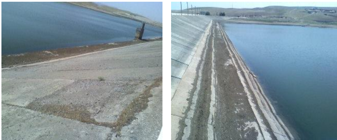
Figure 1. Defects in the pressure slope of the dam
