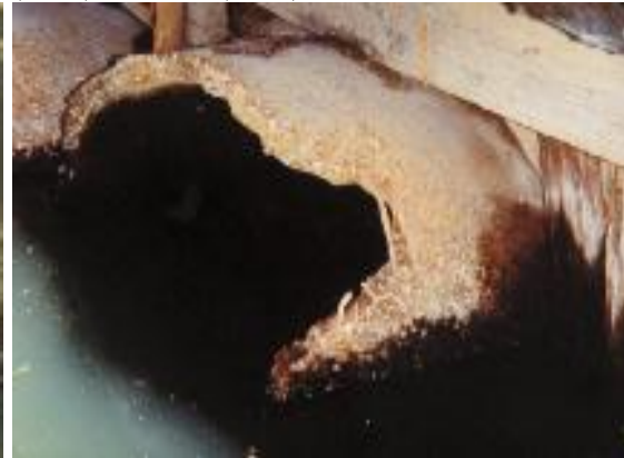
Figure 8b: Corrosion of Sewage Pipes/Concrete
