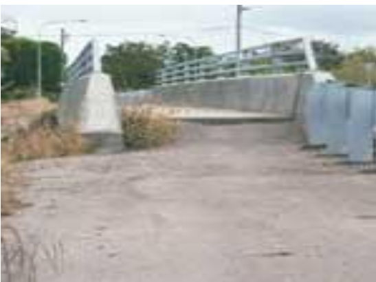
Figure 9: Collapse of Landfills
