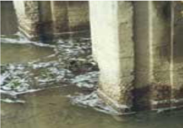
Figure 8a: Corrosion of Concrete Pillars and Steel.
