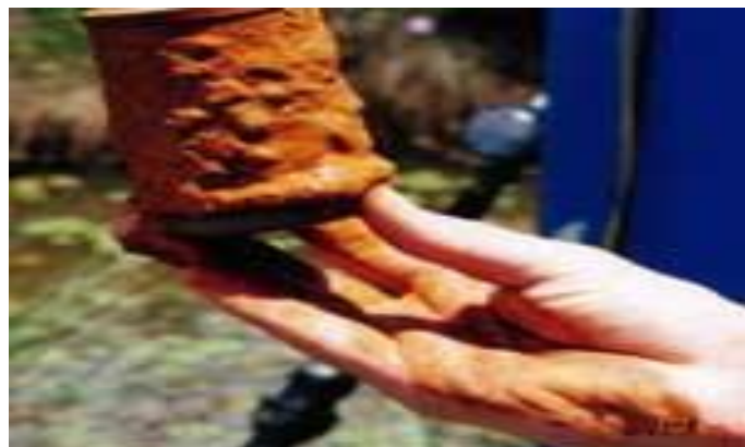
Figure 10: Blocked Perforated Plastic Pipe
