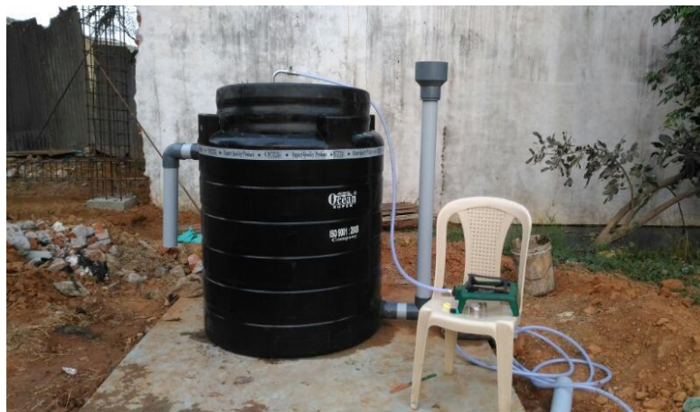
Fig.11 Biogas Plant at SSE Boy's Hostel Mess
